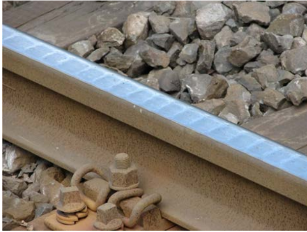
FIG. 1. An example of short-pitch corrugation in light rail systems.
