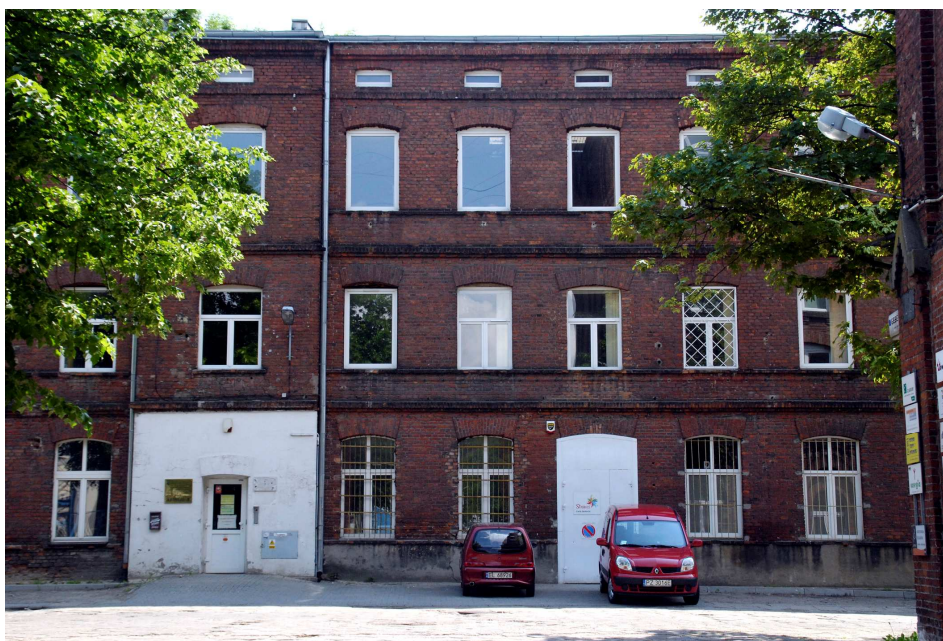
Fig. 4. An example of a building where an uncontrolled replacement of window frames led to the complete loss of the original aesthetics. Photo A. Kurzac
