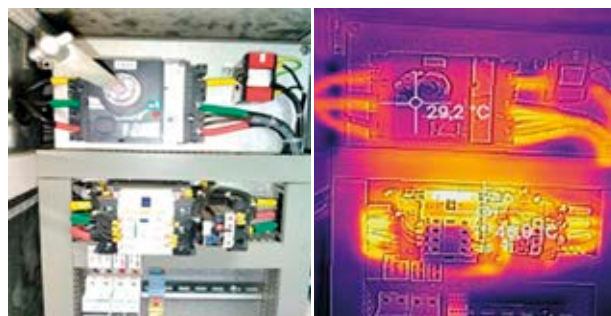
Figure 7. Visible light image (left) and thermal image (right) of an electrical circuit in the pumps
