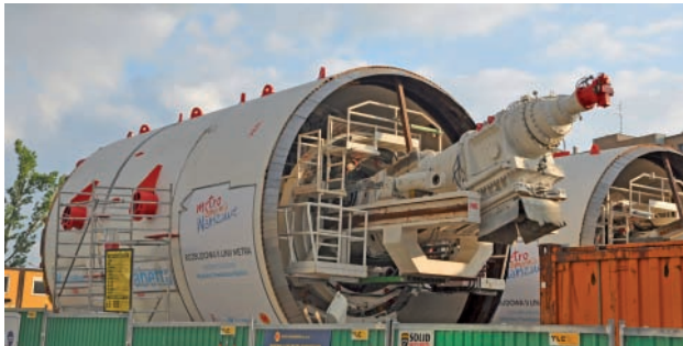
Fig. 18. The Elisabetta TBM in the area of the future Bemowo station (13/06/2020) [photo M. Graff]
