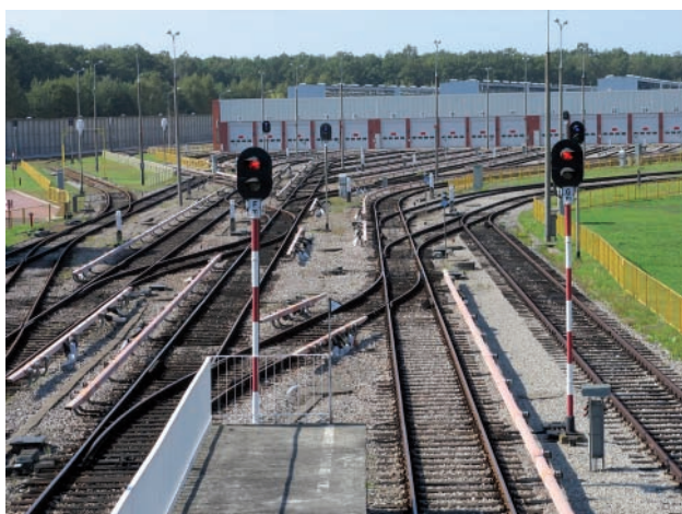
Fig. 27. The Kabaty technical and holding station (STP) (23/09/2006) [photo: M. Graff]
