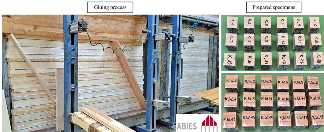
Figure 6. Process of gluing load-bearing beams in ABIES Poland Ltd. and prepared specimens
