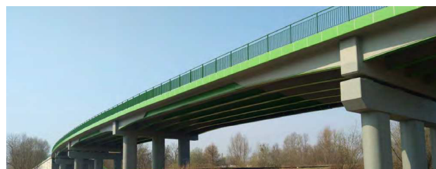
Figure 2: Bridge in Elbląg using both steel and concrete webs in the girder [4, 5].
