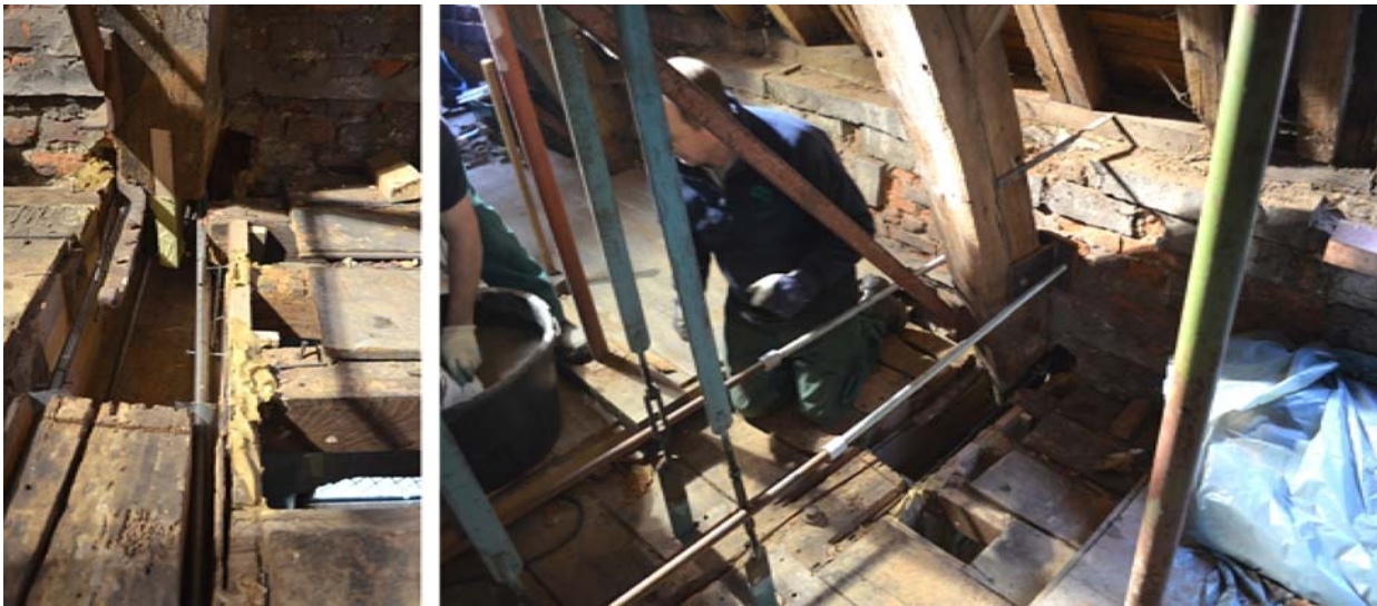
Fig. 3. Example of resin repairs for notched joint: the end beam is cut off and a new ends is poured in epoxy resin. Restauration of the Old castle of Ecaussines-Lalaing, Belgium
