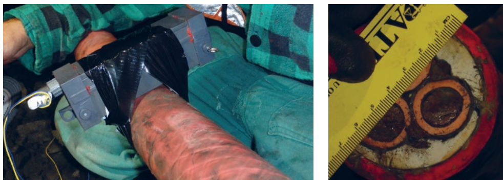
Fig. 22. 150 mm long DIOPLEX™ 400 charge attached to the sheathed mining cable \varnothing 75 mm filled plastic explosive RIOPRIME 25 weighting 60 gr Source: Private gallery (P. Hałys).
