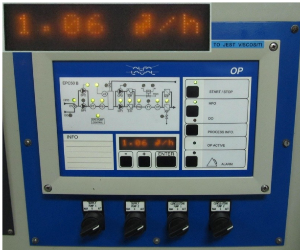
Fig. 2. Fuel flow meter showing current fuel consumption of 1.06 \text{ m}^3/\text{h}
