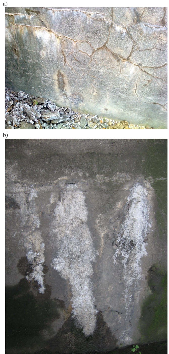
Fig. 4. a) Flyover pier with ASR symptoms, b) gel exuding on the surface of concrete
