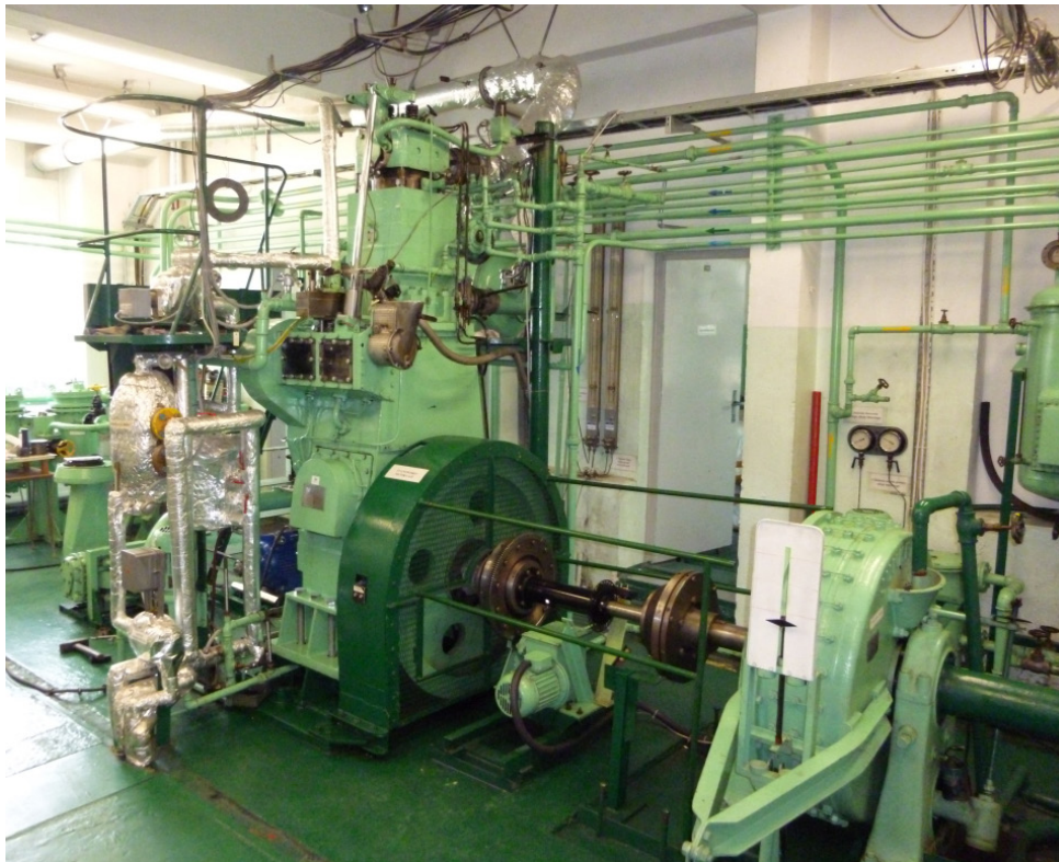
Fig. 1. Test stand with engine L-22 and water brake
