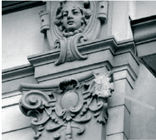
Fig. 9. The picturesque elements from Roman cement on the top part of façade of building. Foto: M.Bevz, 2009.
