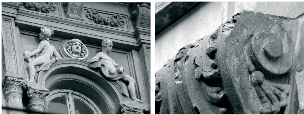
Fig. 13-14. The details from Roman cement on the elevation of the Opera art laboratory. Foto: M.Bevez, 2009.
