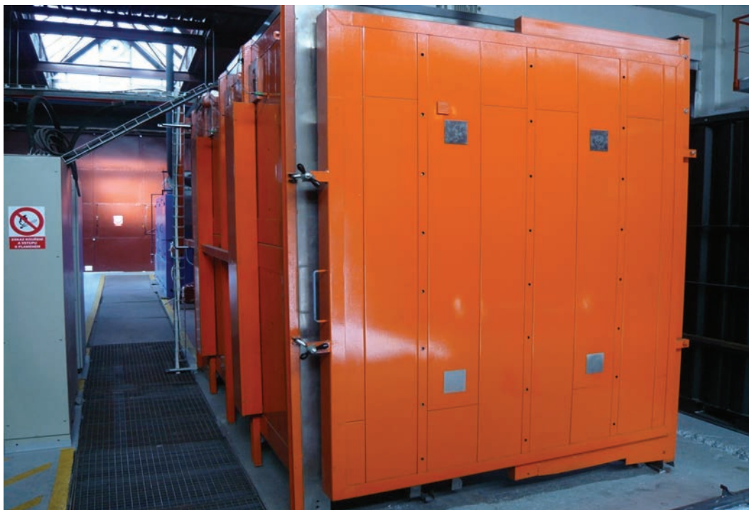
Fig. 2 Pyrolysis plant PTR 1000 (HEDVIGA GROUP plc) – thermal module [10, 11]
