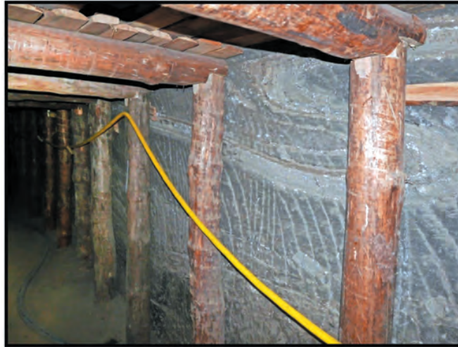
Fig. 2. Baum longitudinal. The area of the planned shaft. Exposure of bronze salts with intergrowths of anhydrite claystones. As of July 2017 [4]
