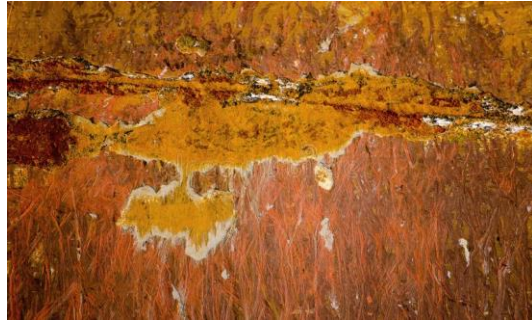
Figure 4. Intensive weld seam corrosion[8]
