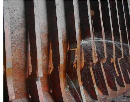
Figure 5. Intensive plating corrosion[8]
