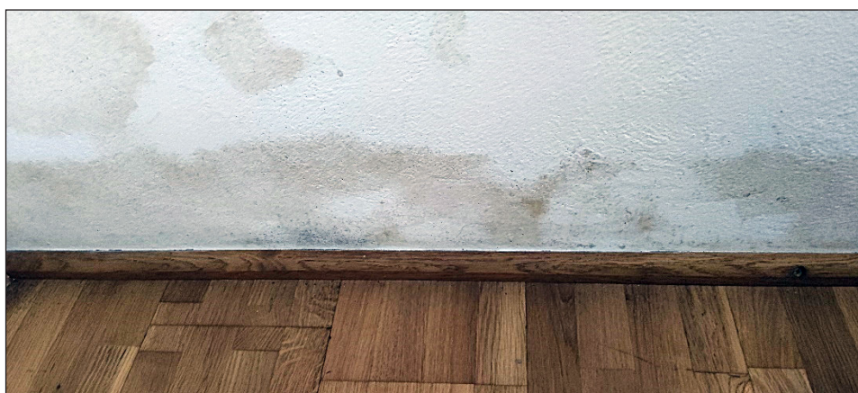
Fig. 4. The dampness of the curtain wall from the inside at the connection with the floor in the analysed object
