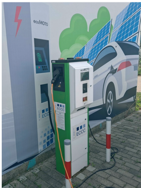
Fig. 6. Appearance of a research charging pole with a maximum power of 22 kW connected to a photovoltaic system
