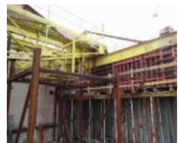
Fig. 11 Construction of a new supporting wall for a historic gantry, own archive, 09.03.2016
