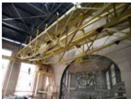
Fig. 7 Historic gantry located in building B2, in the former control room and switchgear before the renovation, 28.06.2016, own archive
