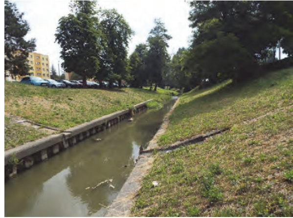
Phot. 6. Reinforced banks and channel (RI). Urban development (SU) (photo L. Borek )
