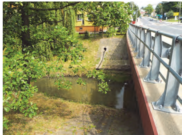
Phot. 8. Intermediate storm water drainage outlet. Reinforced banks of concrete slabs (RI) (photo L. Borek )
