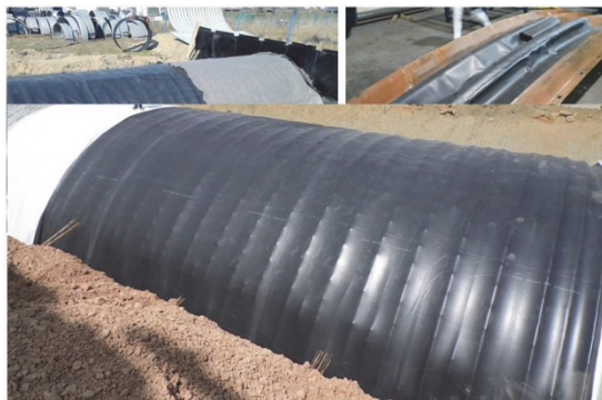
Fig. 29 EPDM geomembrane placed on super-core structure. Railway tunnel in Algeria. Span of circular structure is over 12m
