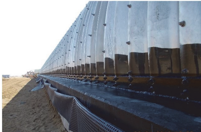
Fig. 9. Performed hydro insulation of external bearing support. Animal overpass PZ-6 over express road S-8 in Poland
