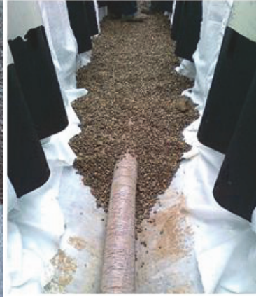
Fig. 15 Drainage performed on intermediate footing. Animal overpass WZ-61C over express road S-5 in Poland
