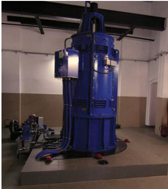
Fig. 2. Tested turbine set in a technical room located in the hydroelectric power plant
