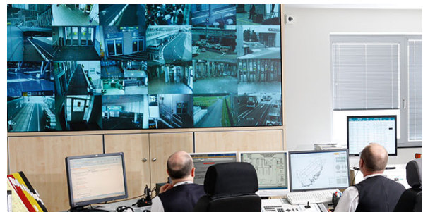
Figure 1. The Flughafen Düsseldorf Security GmbH – Safety and service first hand
