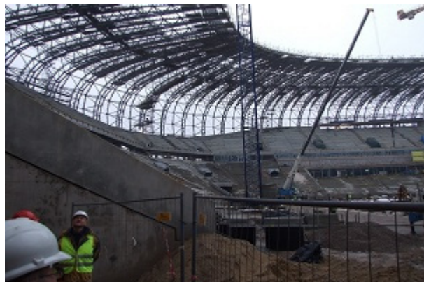
Fig. 4. View of the girders from the side of the pitch - the second stage of assembly.
