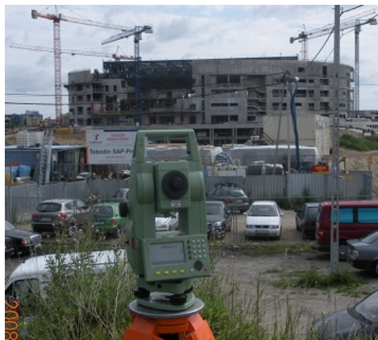
Fig. 2. View of Hall ERGO-ARENA under construction on the administrative border of Gdańsk and Sopot.
