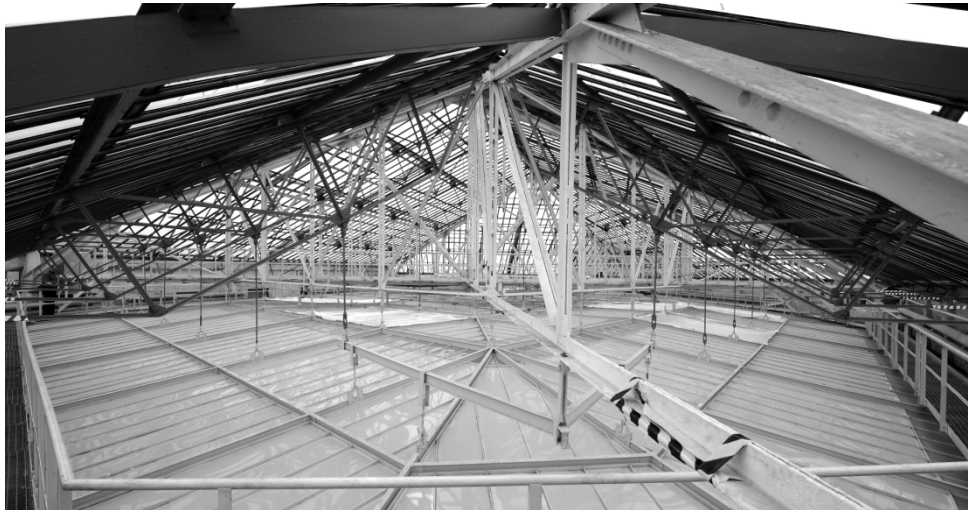
Fig. 1. Photography of a steel construction of the roof at WUT Main Hall.
