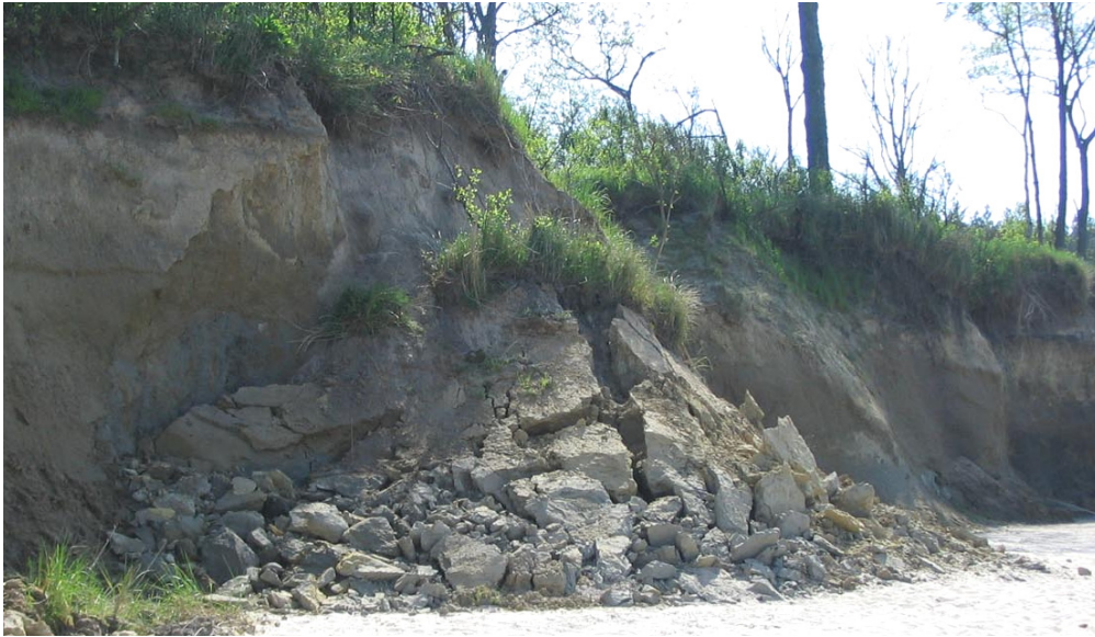
Fig. 7. Landslide caused by abrasion – Pleśna 12.05.2008 r.
