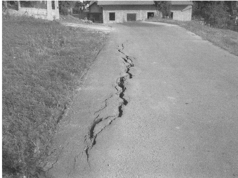
Fig. 3. Damage on a road in the vicinity of the church of St. Mary in Granesina.
