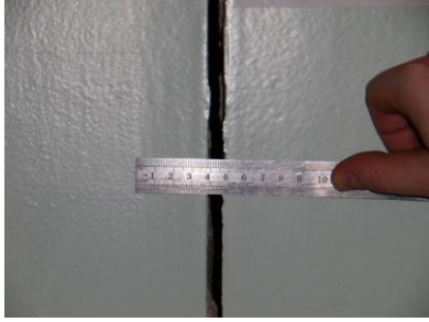
Fig. 1. Cracking of a wall: Engineers of Shaping an Environment building.
