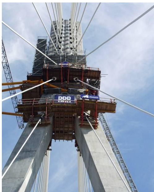
Fig. 3. The Świętokrzyski Bridge - platforms on the pylon serving for assembly of the bridge carrying ropes.
