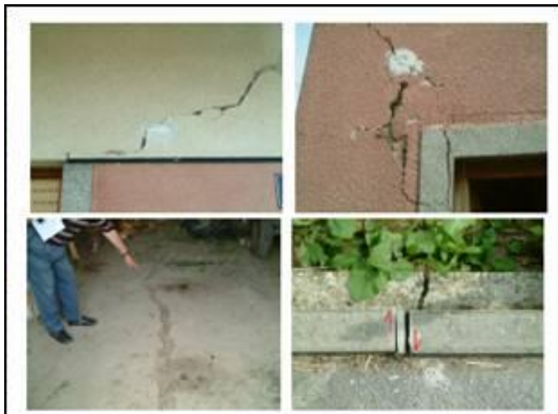
Figure 3. Examples of damages on houses in the epicentral area near Zagreb.
