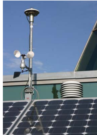
Figure 2. LB-741 – field weather station
