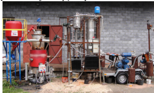
Fig. 4. The complete installation for the gasification of dried sewage sludge and purification of the produced generator gas
