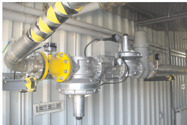
Fig. 4. The gas path of the GE JENBACHER JMS 316 GS-B.LC Biogas Engine
