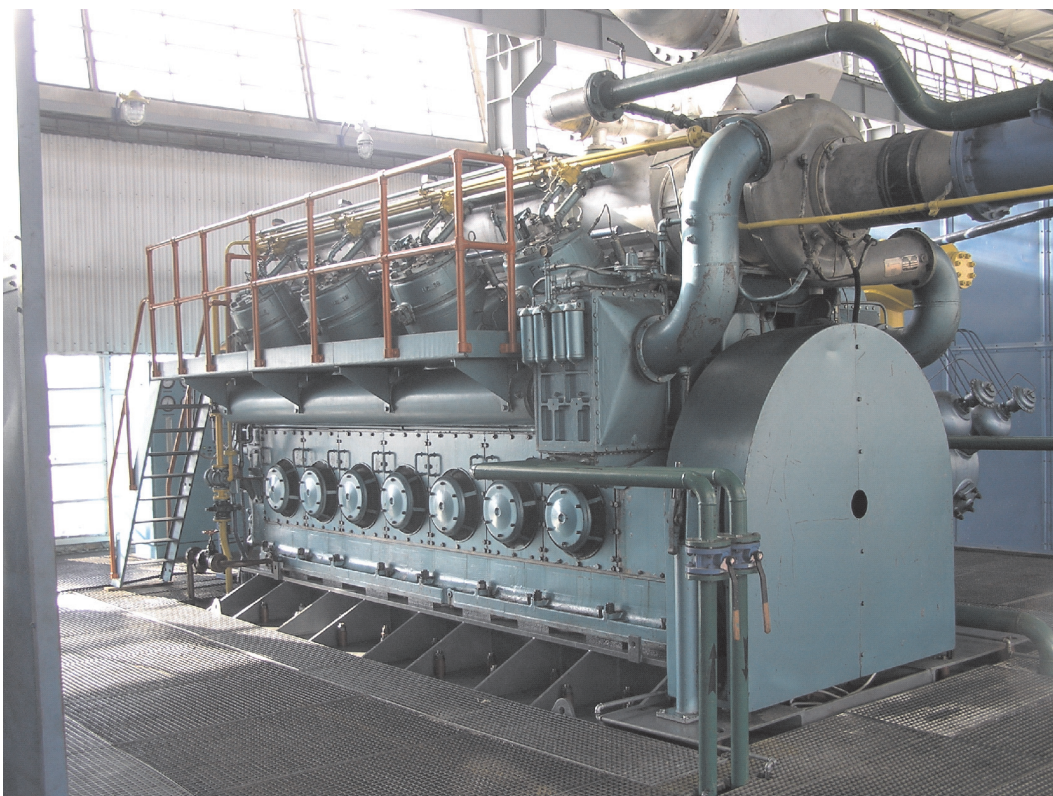
Fig. 1. General view of the Integral Engine-Compressor Cooper Bessemer GMVH-8.
