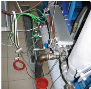
Fig. 10. Picture of the thermoelectric generator mounted on exhaust system of self-ignition engine
