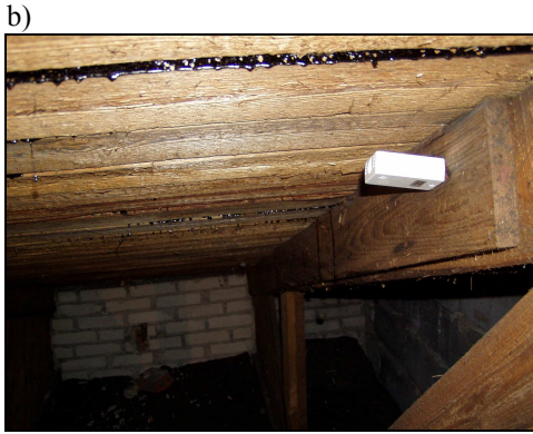
Fig. 4. Sensors mounted at the site: at the insulation layer (a), and at the roof surface (b).
