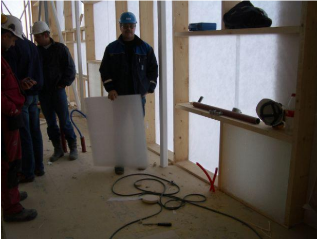
Photo 2. Moniflex wall under construction, overcast sky. The man at the middle holds a 5cm thick moniflex sheet.
