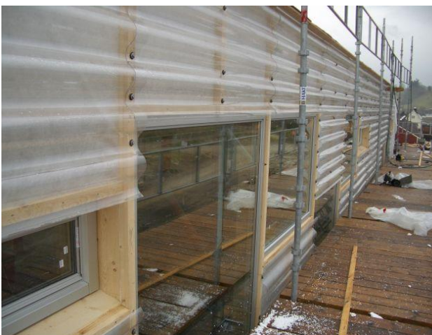
Photo 4. Translucent moniflex wall seen from outside, two types of window detail; for open able window to the left, for fixed window to the right, overcast sky.
