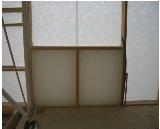
Photo 1. Translucent moniflex wall under construction seen from inside, overcast sky. 20 cm moniflex in the midfield; translucent wind cover in the adjacent sections.
