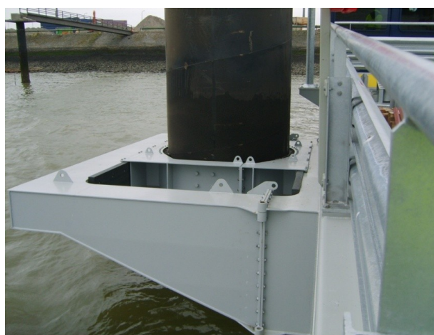
Fig. 8. Pontoon ramp pile anchor with possible ramp movement
