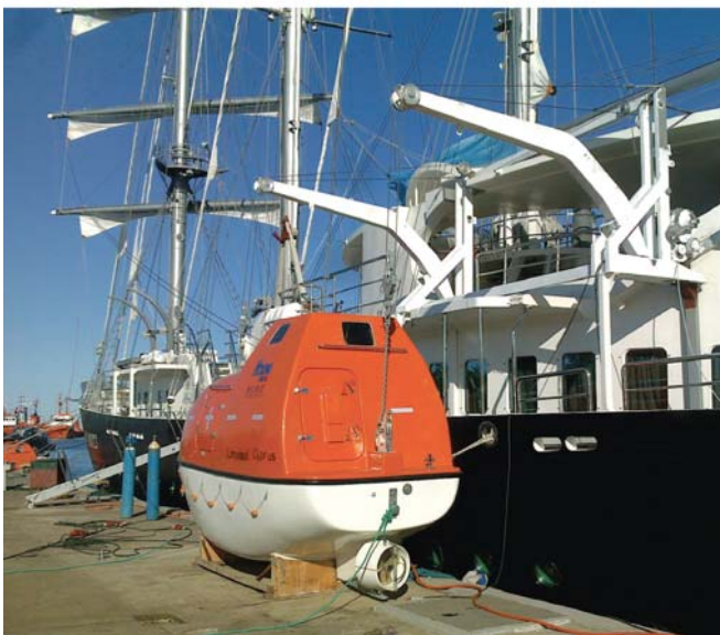
Fig. 4. The life boat davits during and after installation of them on a sailing passenger ship.
