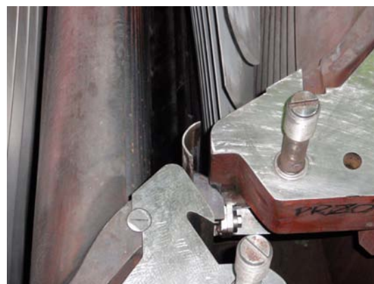
Fig.22. The ring placed inside 225 MW turbine
