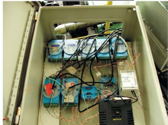
Fig. 8. System transmitting and recording the data collected from sensors
