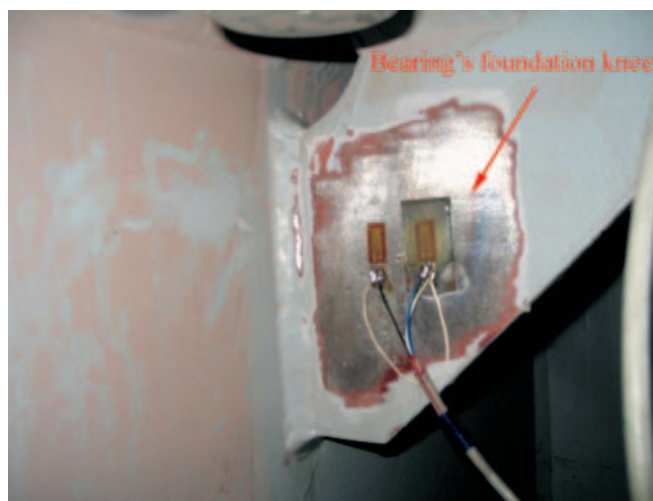
Fig. 4. Stress measurement of bearing's foundation knee
