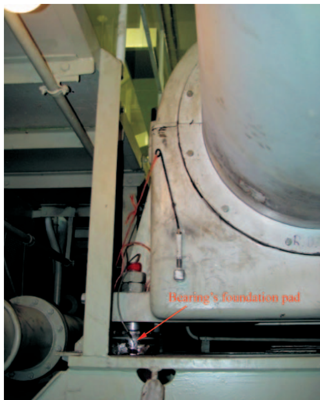
Fig. 3. Stress measurement of bearing's foundation pads
