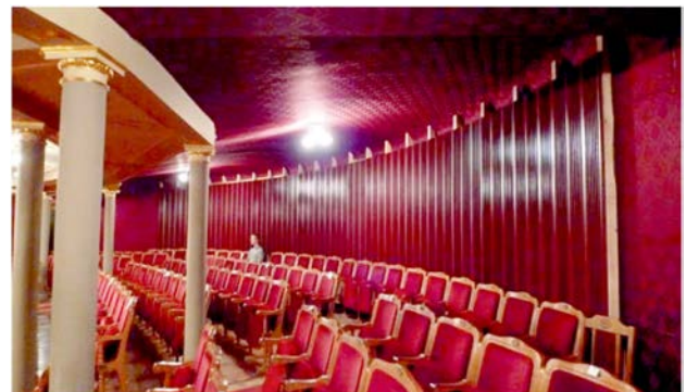
Fig. 10. A view of the semicircular back wall behind the underbalcony space in the Lviv Opera House after installation of diffusion panels.
