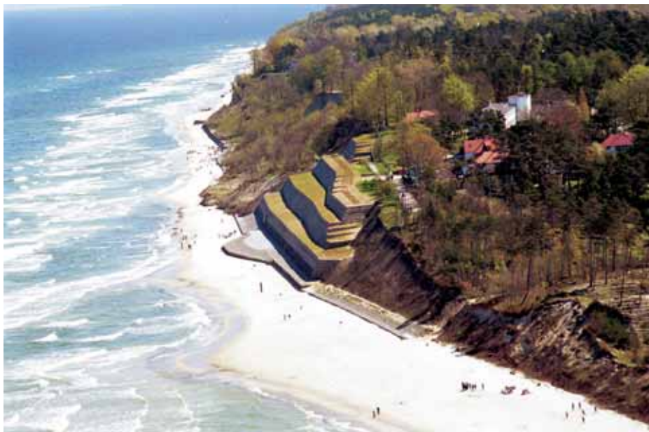
Fig. 7. Stepped stony wall protecting of the Jastrzębia Góra cliff's slope, built in 2000, and new landslide behind the wall (Photo. by P. Domaradzki, 2001)
