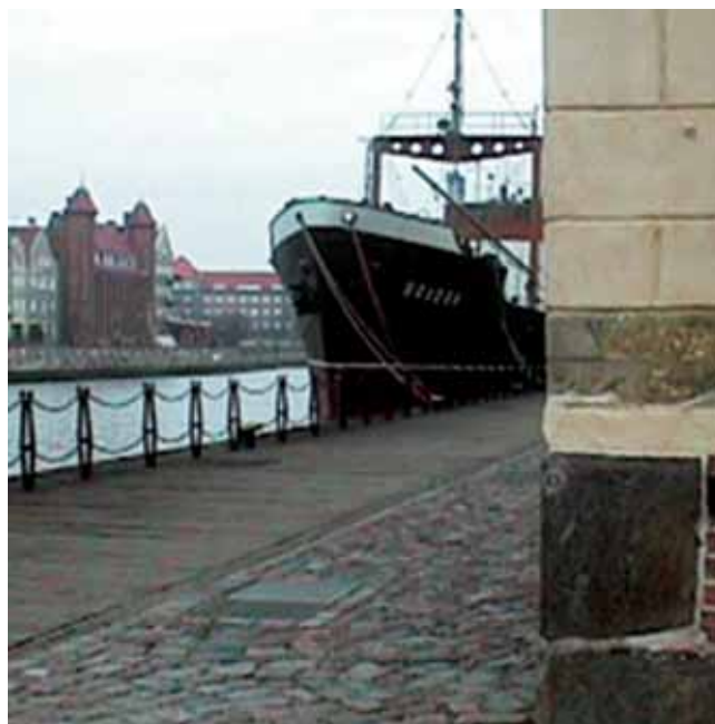
Fig. 9. Mark of the highest water stand on the wall of old granary, indicating 3.36 m above the mean sea level
