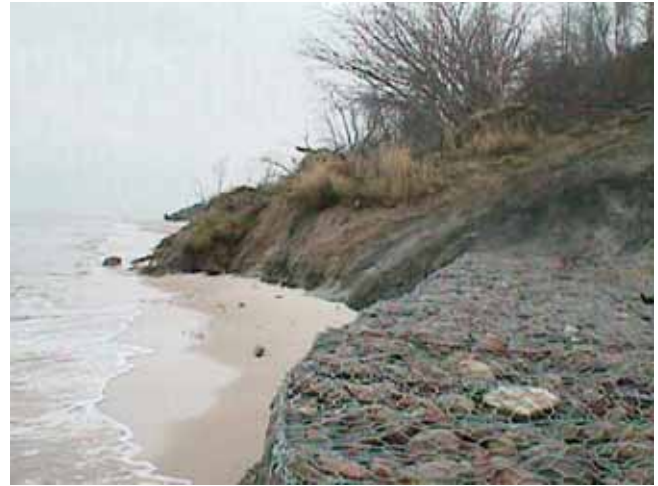
Fig. 6. Seawall built in 1994 for protection of the cliff, partly destroyed by landslide in January 1999 (Photo. by Sz. Uścińowicz)
