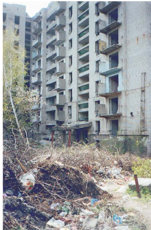
Fig. 3. Abandon 14-storeyed dwelling house, deformed as result of landslide activation
