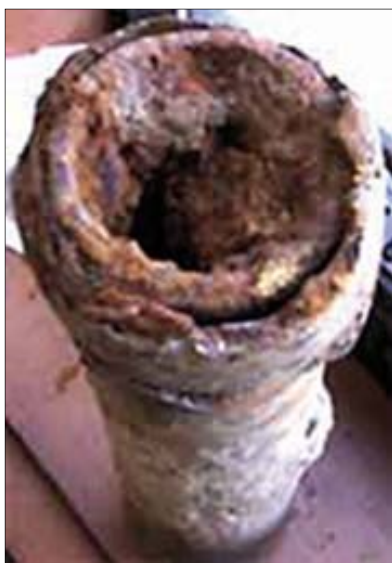
Fig. 3. Typical scale found in pipes in the field.
