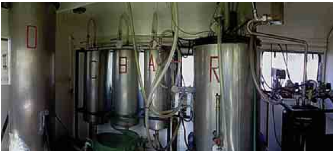
Fig. 1. A panoramic photograph of a mobile biodiesel production plant constructed inside the body of a Star 266
