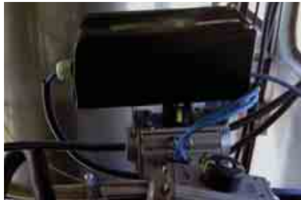
Fig. 4. A cold-water valve with a positioner
