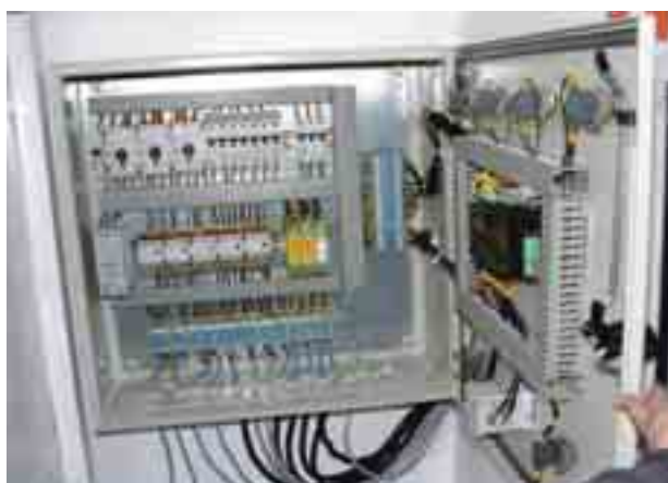
Fig. 3. A control cabinet with electrical protection elements and a PLC-HMI controller installed on the cabinet door
