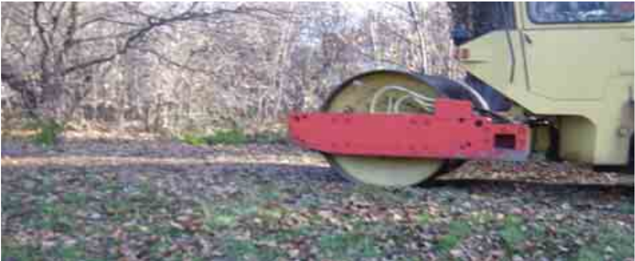
Fig. 1. A photo of a vibrating roller during its rides at the times measurements
