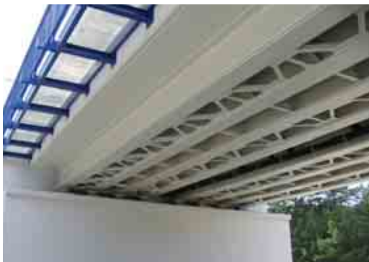
Fig. 1. The modernized viaduct No. KNI 140 070 composed of two separate spans, located at the PCM Line, Poland. Bottom view on the main beams and bracing
