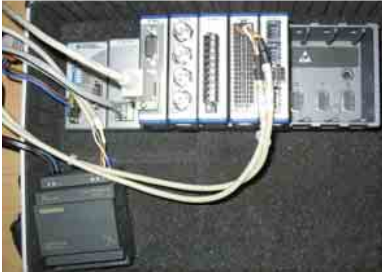
Fig. 6. View of central control module
