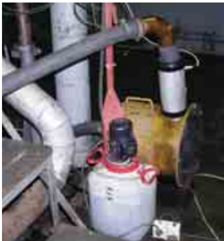
Fig. 7. The equipment of the research stand to measurement of blowthrough to the crank case
